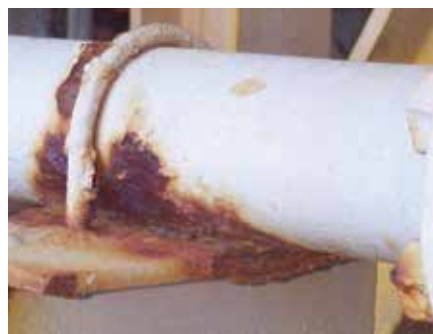
Above: the result of crevice corrosion on a pipe. Trapped moisture has caused wall loss that could result in catastrophic failure.
